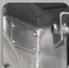
Interlock safety switches on doors
